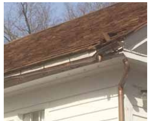
Crushed gutter and roof damage
