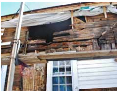
Moisture damage in the west wall
