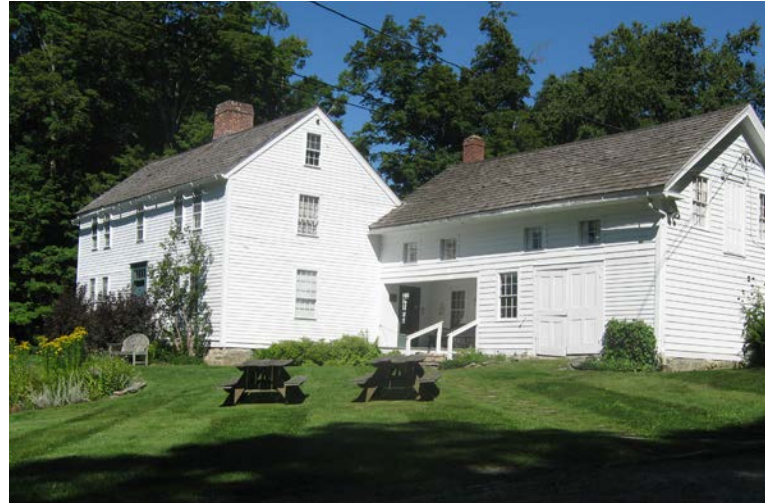
By 2014, the gable overhang is gone, the exterior is white, the porch open. The cedar shingle roof is curling and cracking and needs to be replaced.
